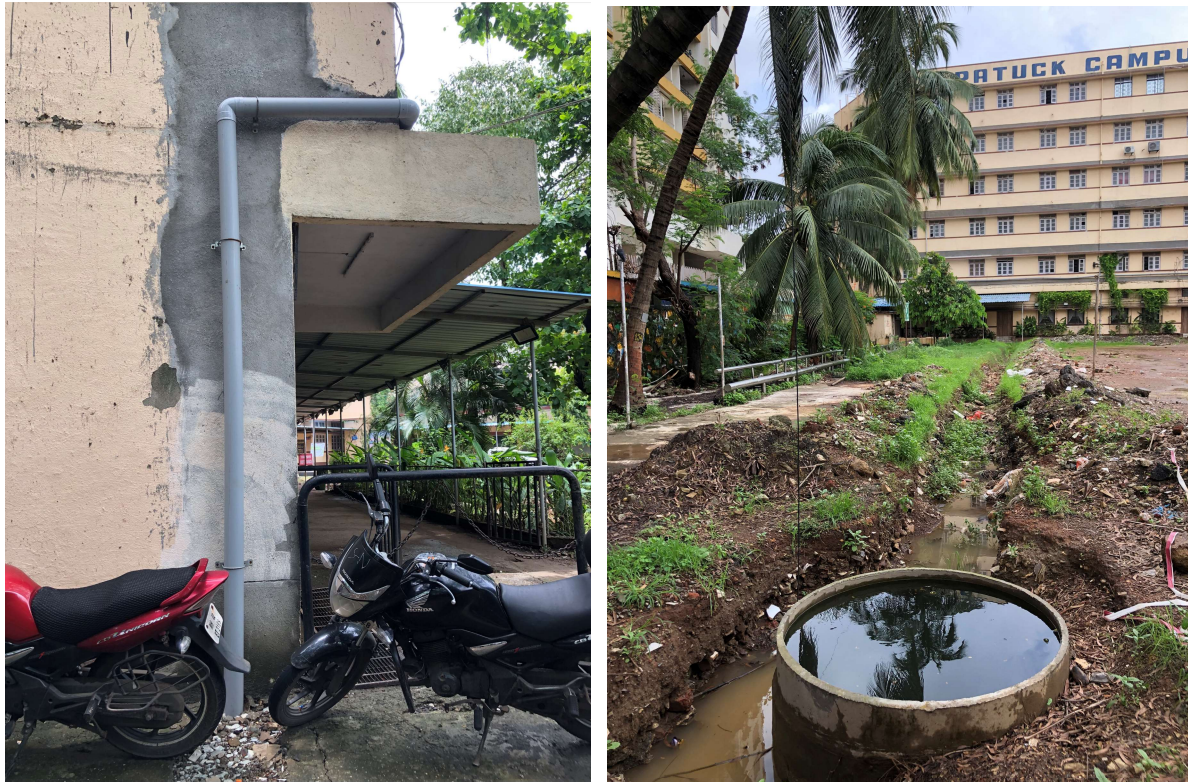
Figure 3: Rainwater harvesting down-take pipe and Recharge pit provision in campus
